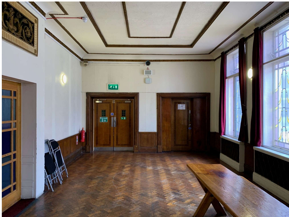
Photo 004 - Photo of far end of the room showing 2 no. original doors, timber panelling, timber floor and ceiling plaster
