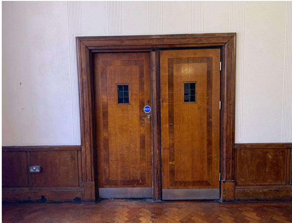
Photo 003 - Original door to Kitchen area and timber panelling along lower section of wall
