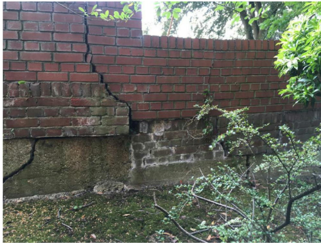
Figure 5 - Cracking to the front party fence retaining wall taken from No. 30
