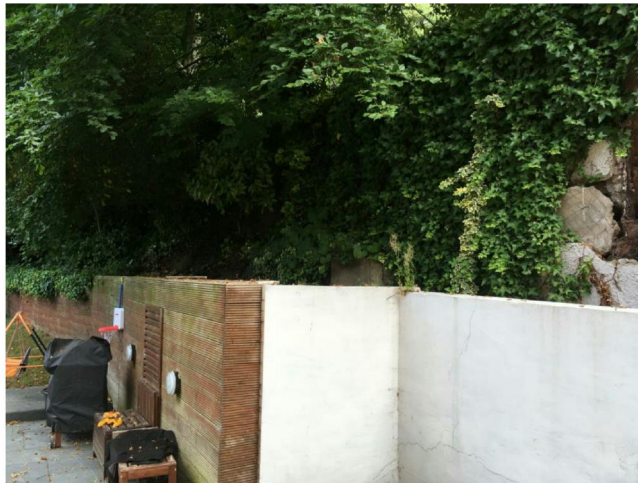
Figure 8 - Garden retaining wall inset from the party fence retaining wall taken from No. 30 facing the garden
