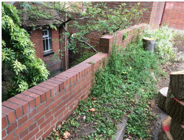
Figure 3 - Retaining party fence wall to front of property taken from No.28 facing the property
