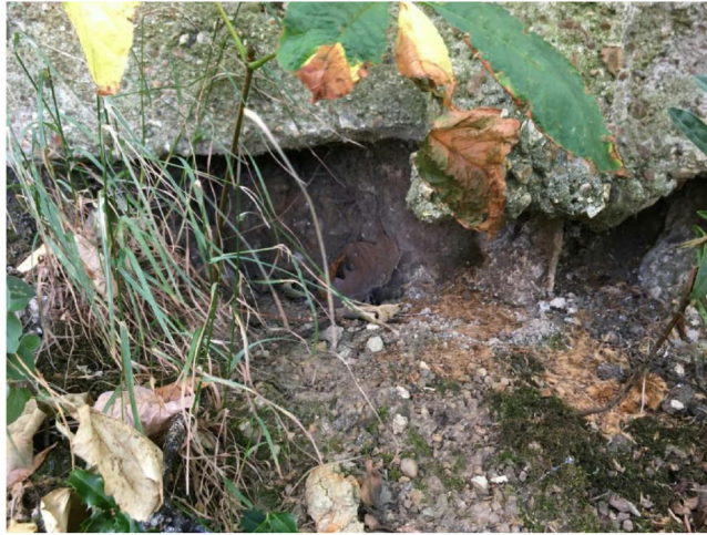
Figure 7 - Evidence of burrowing beneath the shallow foundations of the party fence retaining wall taken from No. 30
