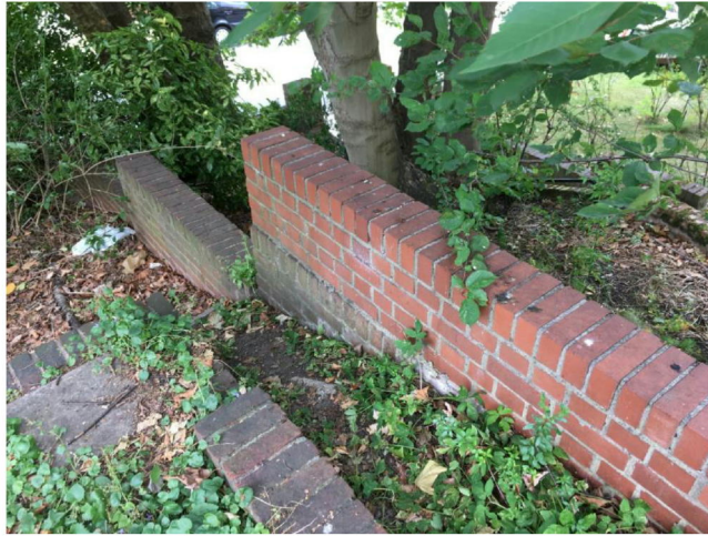
Figure 2 - Retaining party fence wall to front of property taken from No.28 facing Redington Road
