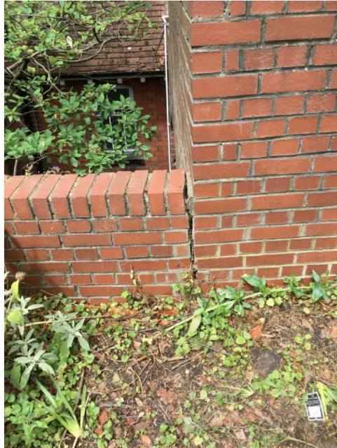
Figure 6 - Cracking at the junction between the party fence wall and party wall to the front of the property taken from No. 28
