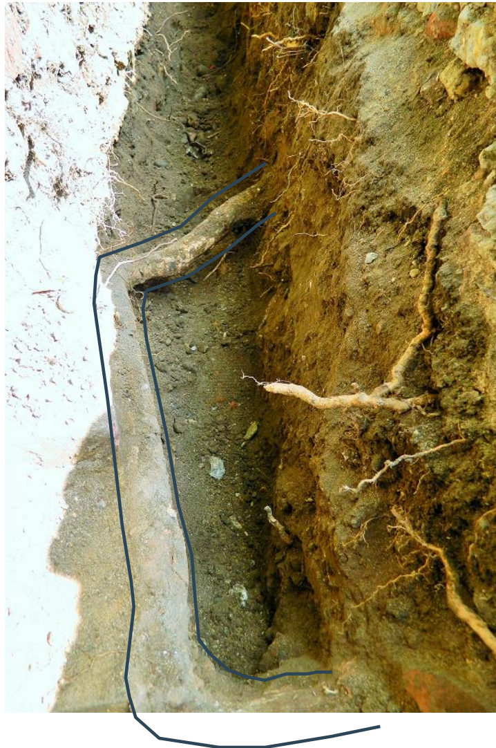
Figure 7. Ash root 50 mm diameter growing out of house-side of exploratory trench and back into the side wall of the trench after 1 m.
