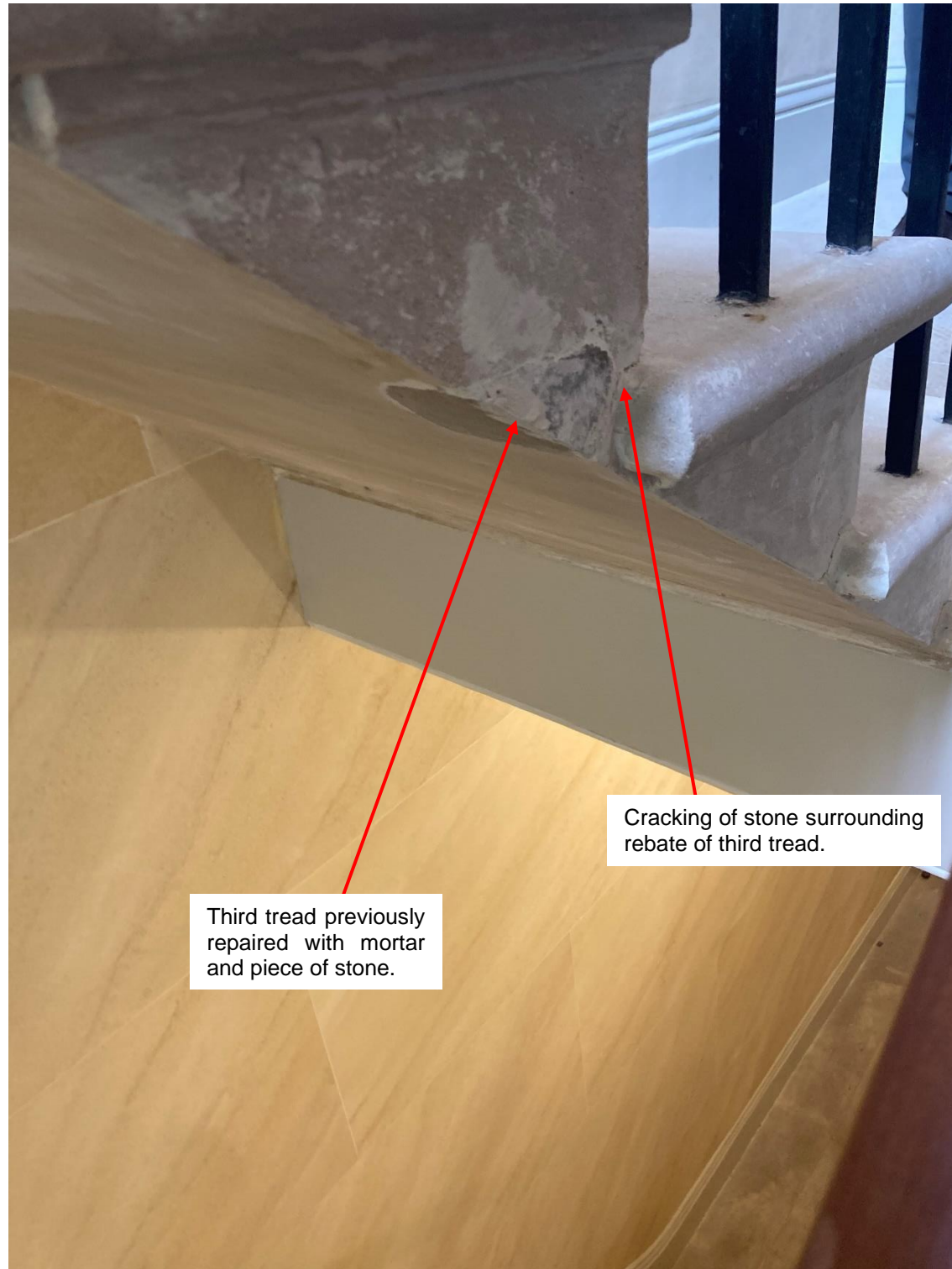
Figure 5: View of third tread above first floor landing showing previous repair and cracking.
