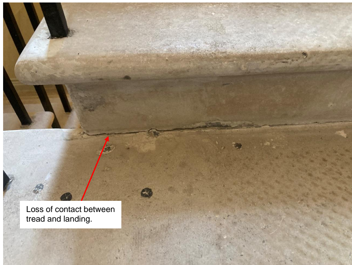
Figure 1: Cracking between first floor landing and first tread above.
