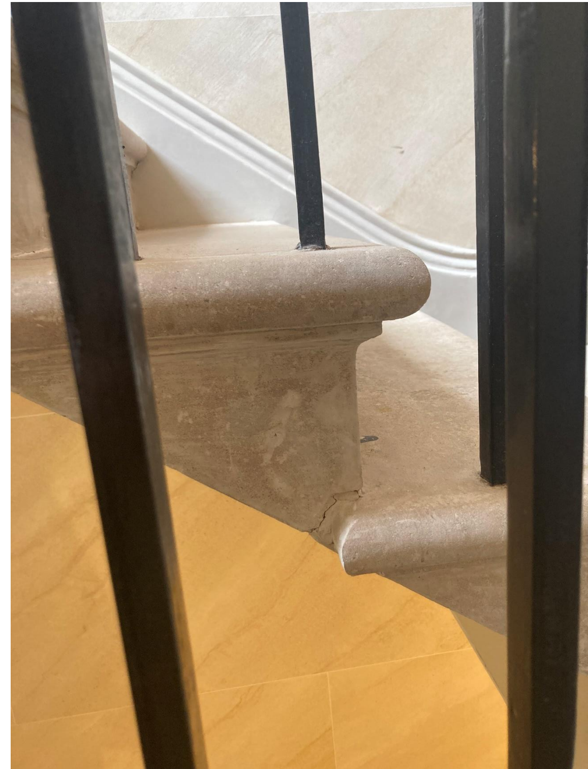
Figure 4: Cracking of stone at rebate construction joint of second tread.
