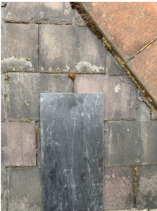
Above: Photographs of sample taken in situ at 25 John's Mews and as presented to Camden Heritage Case Officer Nick Baxter on 03.10.22
