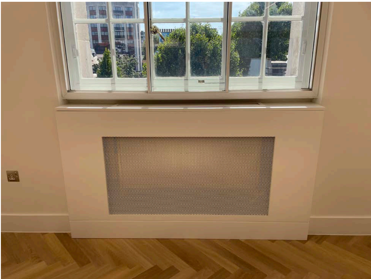
Radiator covers at 3rd floor level. Matching radiator covers proposed at 6th floor level.
