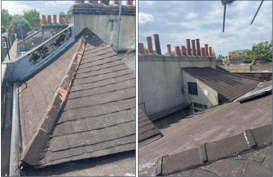
Figs 10 and 11. Details of the roof, showing failure of the Turnerising and deflection exacerbated by the additional weight of the bitumen coating
