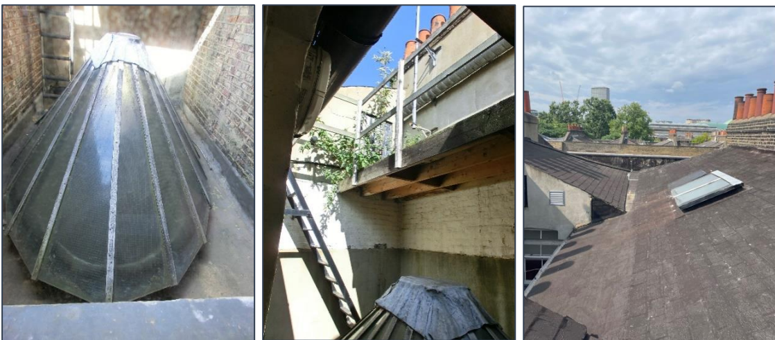
Fig 7 (left). No. 6, roof lantern. Fig 8 (centre). No. 4 roof with metal stair and timber walkway. Fig 9 (right). Slates covered with bitumen (Turnerised)
