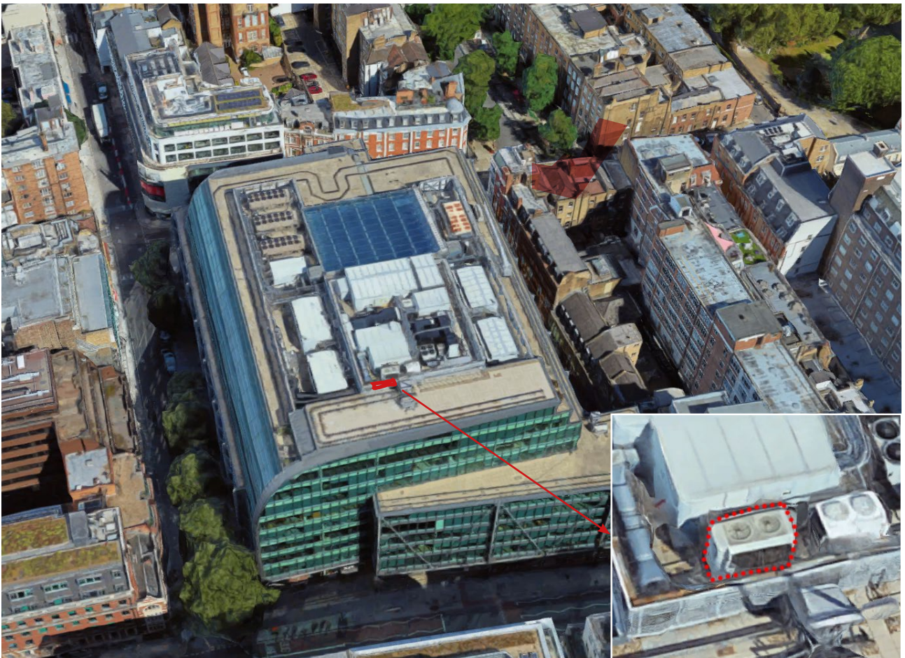
Bird-eye photo showing in red proposed location for the new condenser units. The space is currently occupied by an old chiller which is going to be decommissioned
