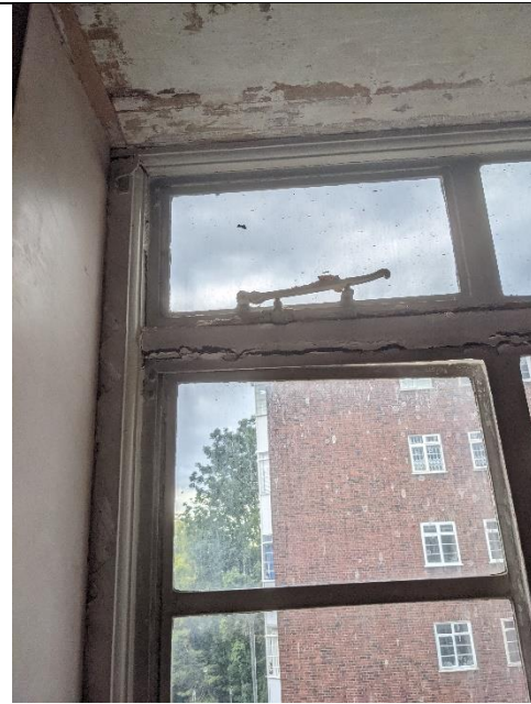
Existing window frame_ Cracked
