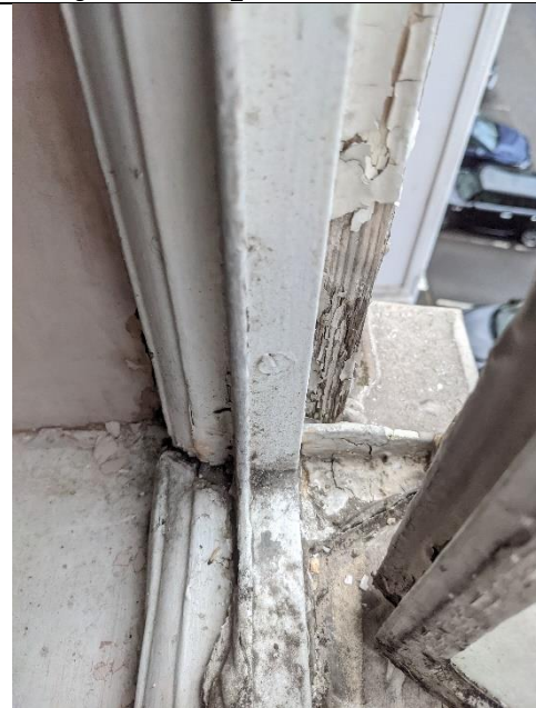
Existing window frame & joint_ weathered and damaged
