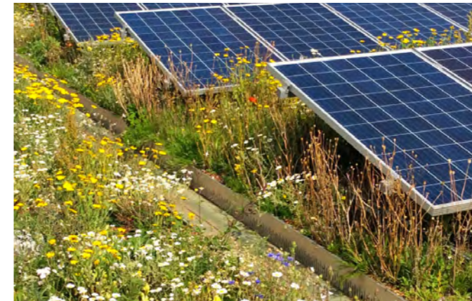
Extensive green roof (Biosolar roof) 0.7
