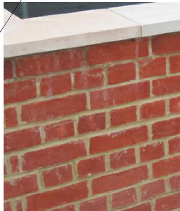
Retaining wall with brick facing and York stone coping. Brick and mortar joints to match existing building.
