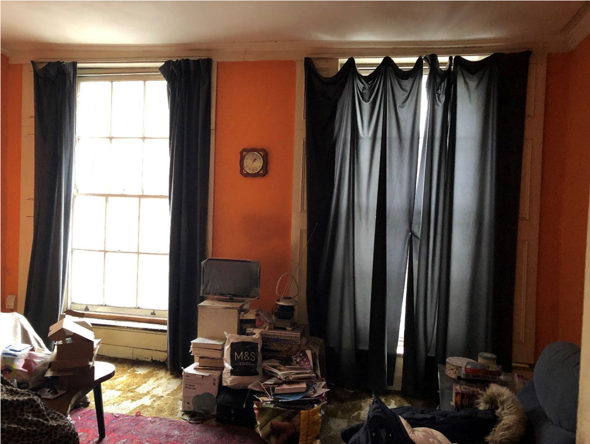
Figure 7 – Internal view of the two timber sash windows to the front of the building at first floor level
