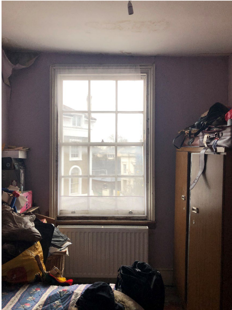
Figure 8 – Internal view of the timber sash window in the left bedroom to the front of the building at second floor level
