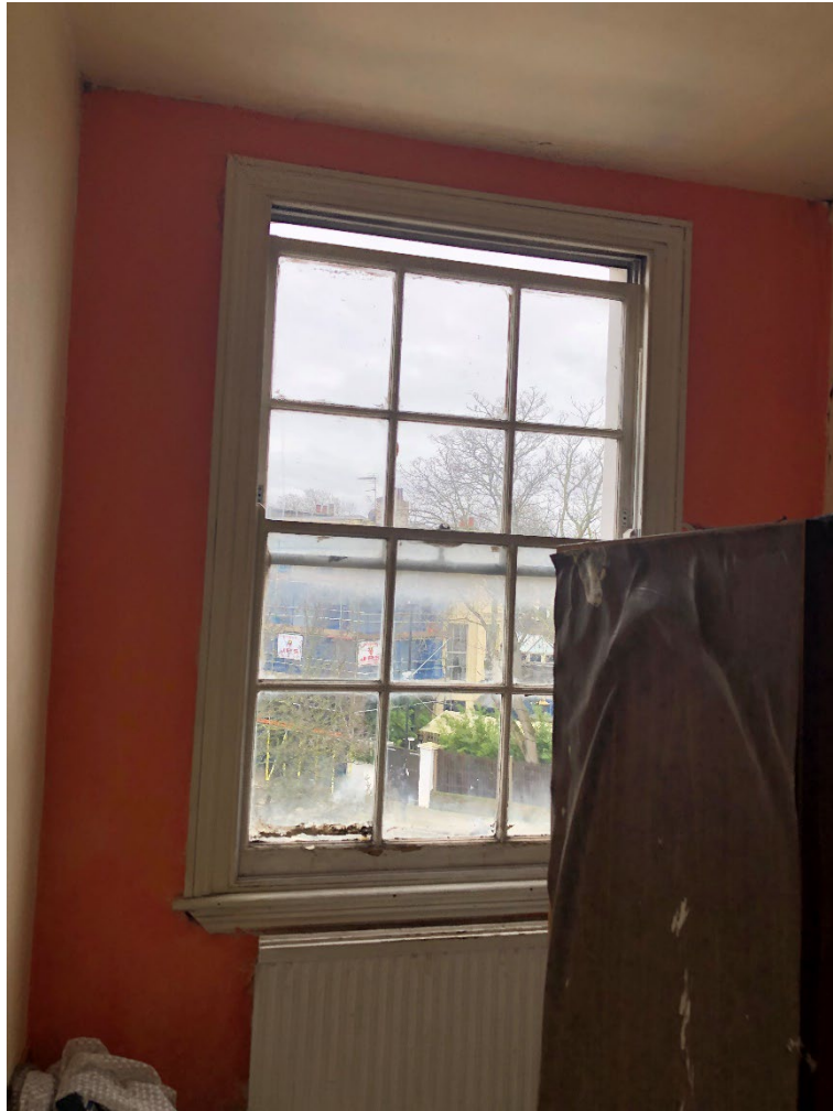
Figure 9 – Internal view of the timber sash window in the right bedroom to the front of the building at second floor level
