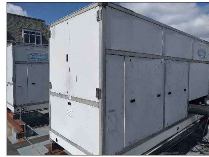
EXISTING CHILLER PLANT ON MAIN ROOF (APPROX DIMENSIONS 3600mm LONG x 1300mm WIDE x 2200mm HIGH)
