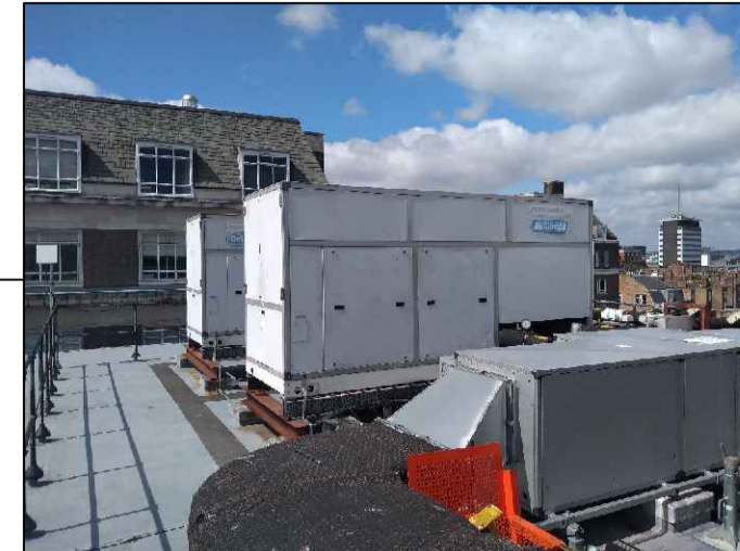
EXISTING AIR-HANDLING PLANT AND CHILLER PLANT ON MAIN ROOF
