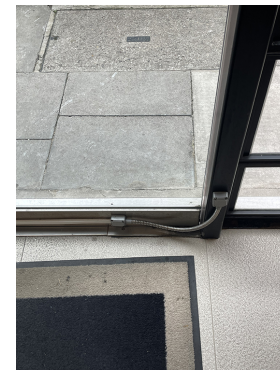
Image 02: Power supply to Lower Mag Lock
