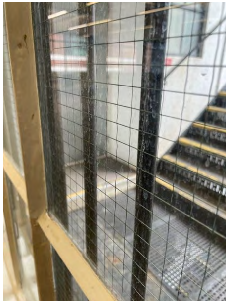
2.1.B -Image of Existing Georgian Wired Glass window that open with 1.8m of an escape route
