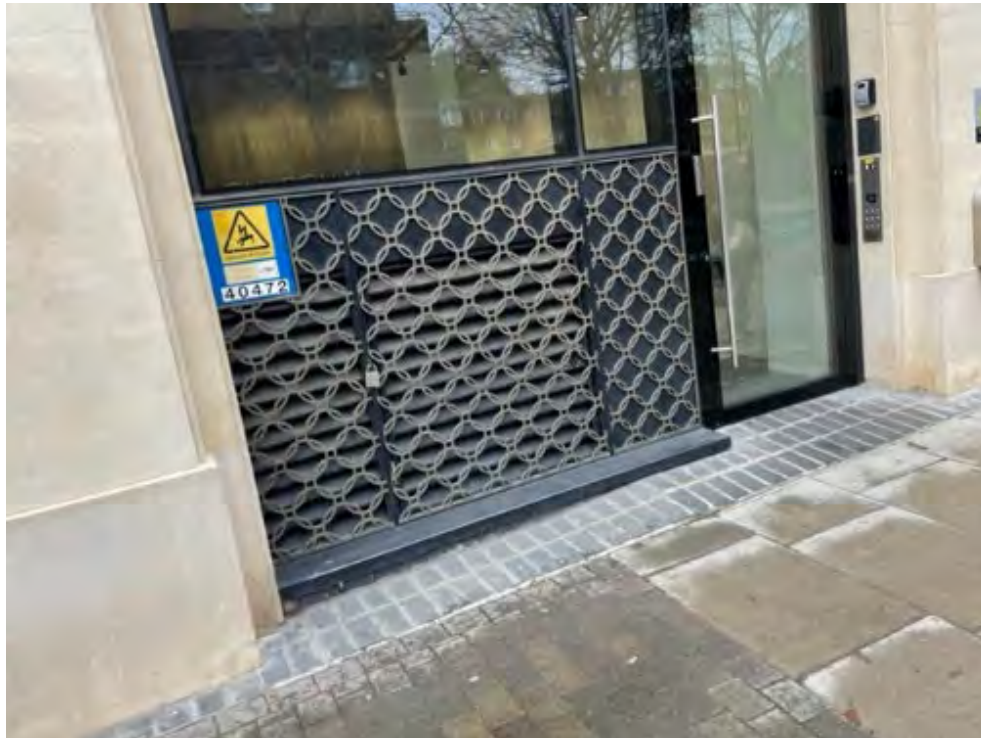
4.1.B Photo of similar louvre cover (note grills to Louvres of Shropshire House would not be faced fixed but recessed into the alcove- refer to HHD dwg no. 253.402 )
