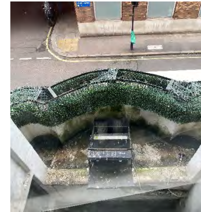
5.1.C Existing Up-lighter (positioned on existing balcony)
