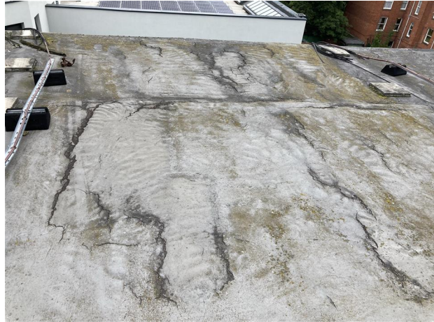
Splits and cracks in the asphalt material will let water by, it has reached the end of its life.
