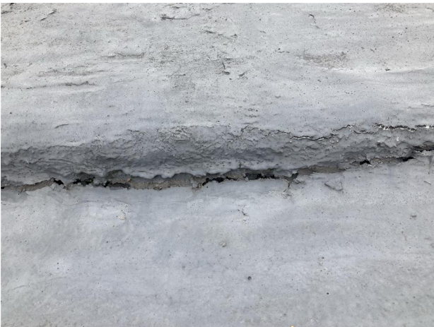
The waterproofing upstand has failed.
