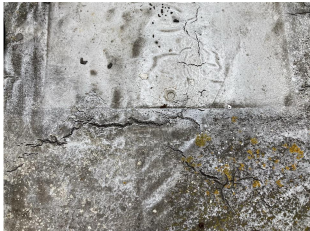
The asphalt has completely deteriorated, it has reached the end of its life.
