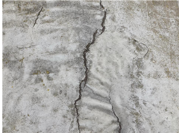
Asphalt has failed.
