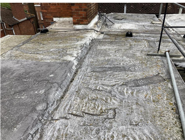
Due to the extent of the poor condition of the asphalt, further repairs are not a viable option.
