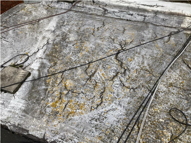
The asphalt covering is badly degraded with splits and cracks.
