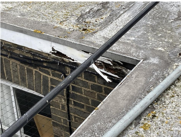
Observation - timber fascias are rotting.
