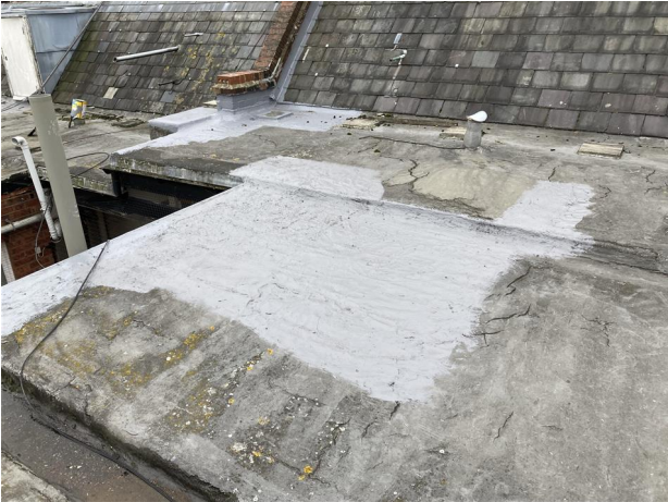
Further evidence of liquid applied remedial coating indicating previous issues and repair history.
