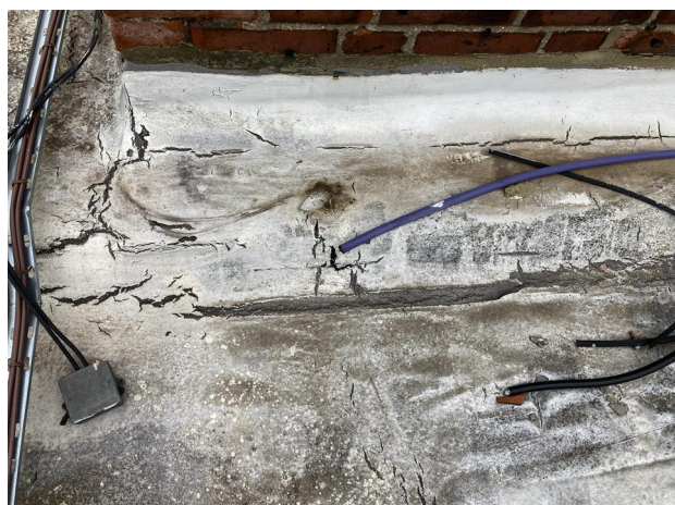
The asphalt material is failing consistently.
