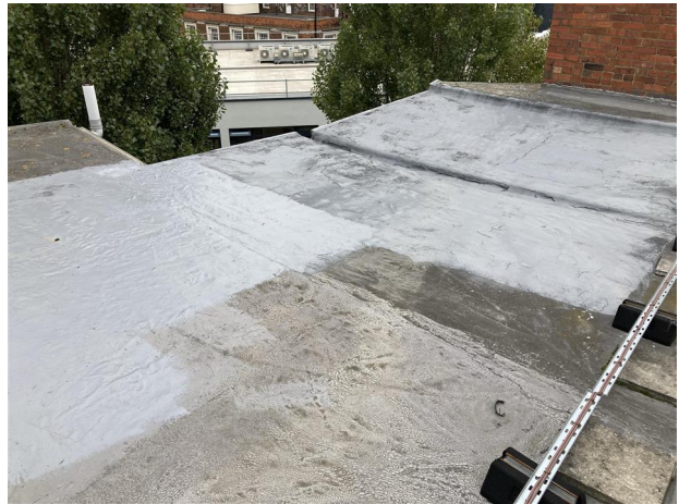
Large area of liquid applied remedial coating indicating previous issues with water ingress and repairs history.
