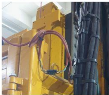
Photo - Drilling Gates Closed - Circuit connected
