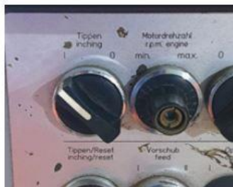
Photo - Forced inching mode - limited movement on drilling controls when gates are open
