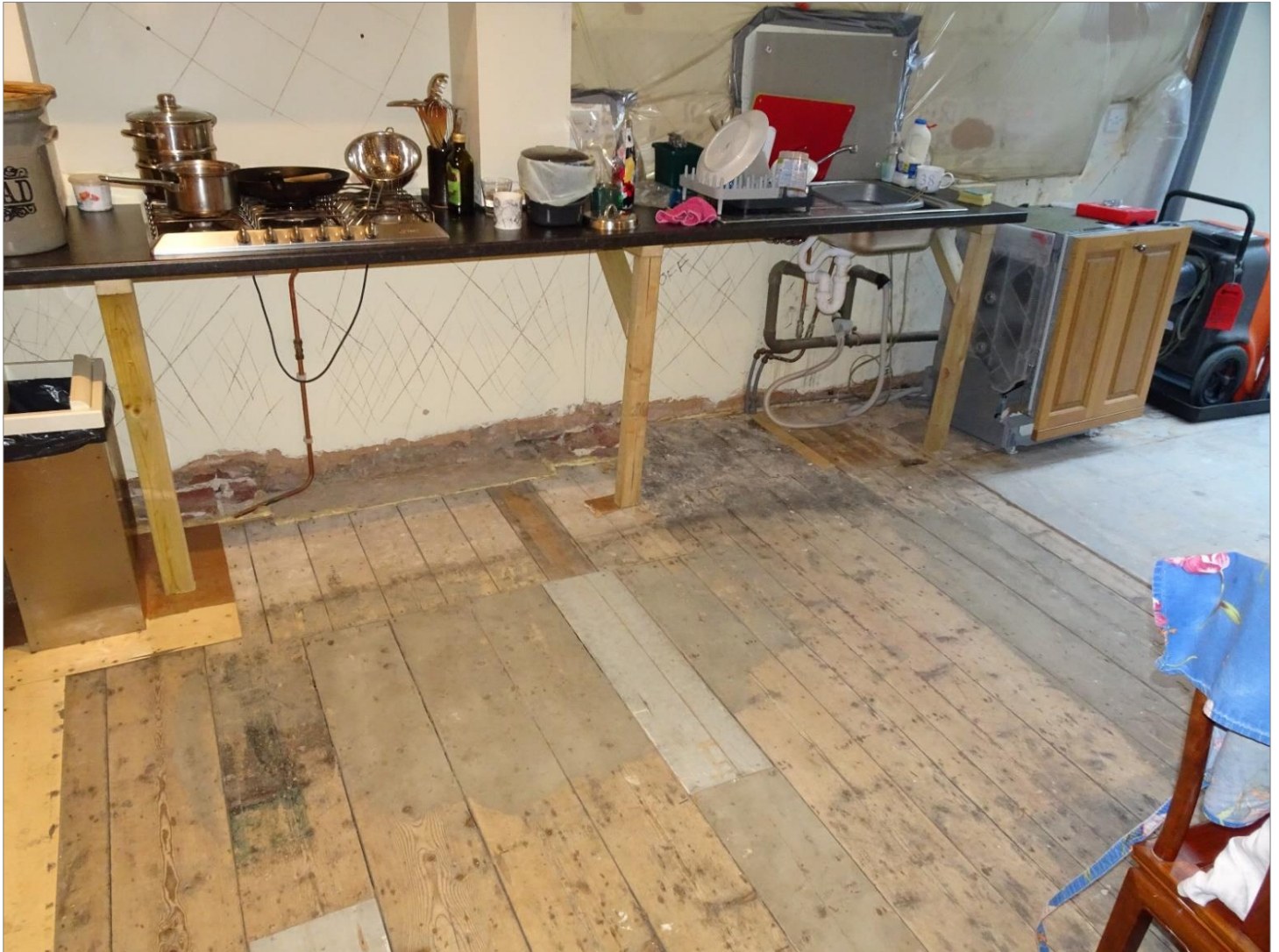
Photograph 1 Kitchen floor - selection of photographs showing patch repairs and non-original floorboards.
