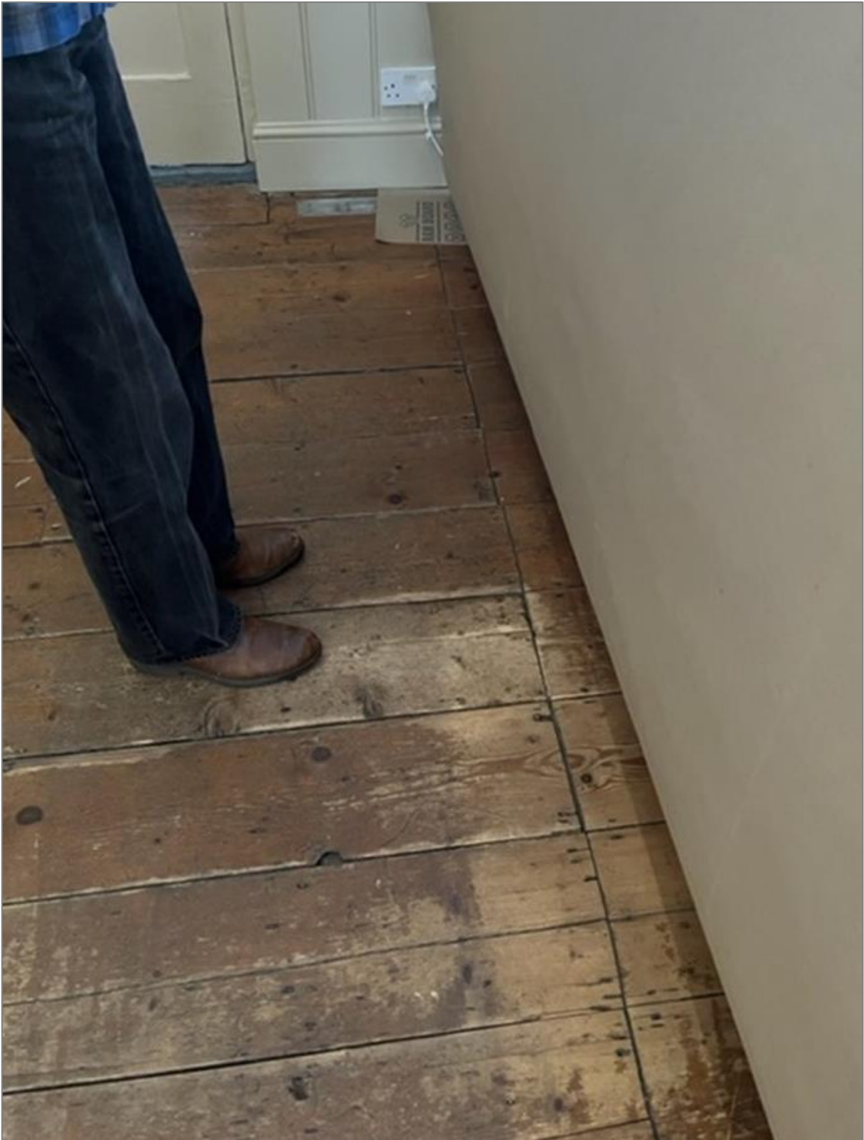
Photograph 8 Cut floorboards requiring repair/possible replacement to dining room
