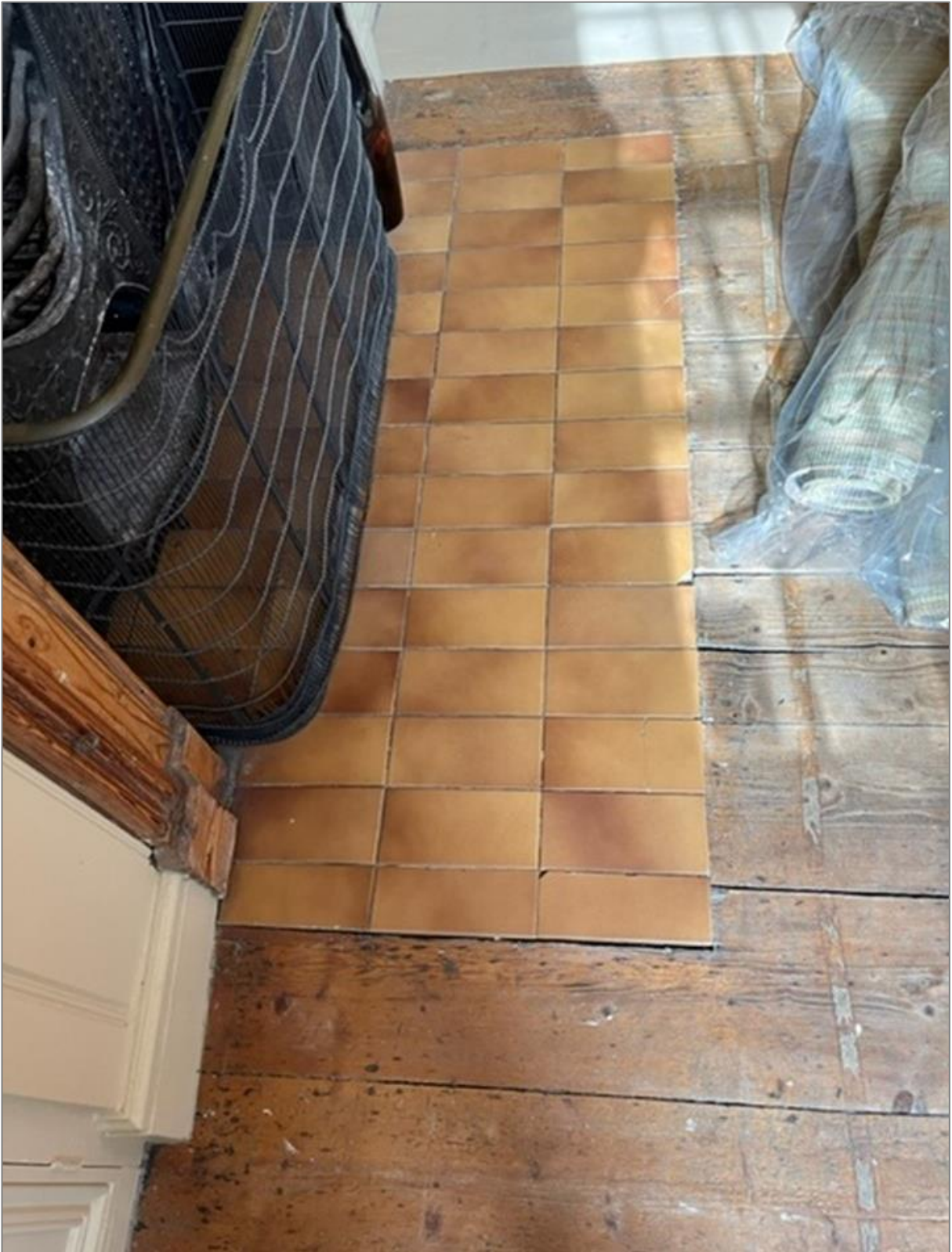
Photograph 9 Cracked non-original tiles to hearth.
