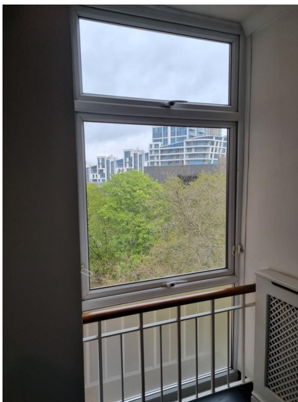
Figure 1 – Existing common lobby manually opening vents
