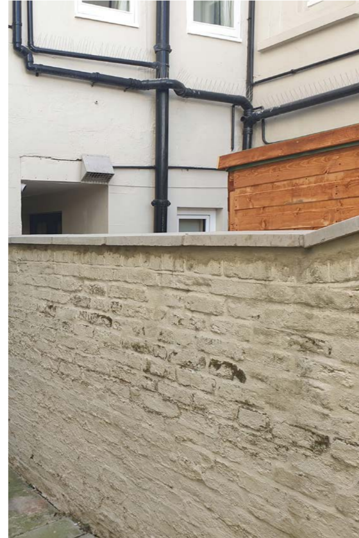
05 | View from No.27 looking over the boundary wall at the lower ground floor with the existing passageway to the rear garden of No. 29
