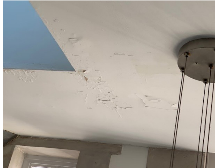
A photograph taken on the 01/08/2022 showing the existing internal condition and water damage to the first floor ceiling.
