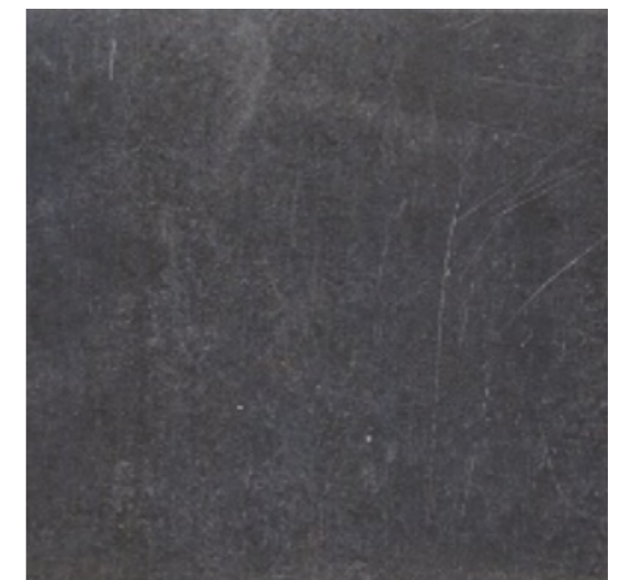
Our proposals are to replace the existing lead flashing with a new Code 5 Lead flashing around the abutments.
