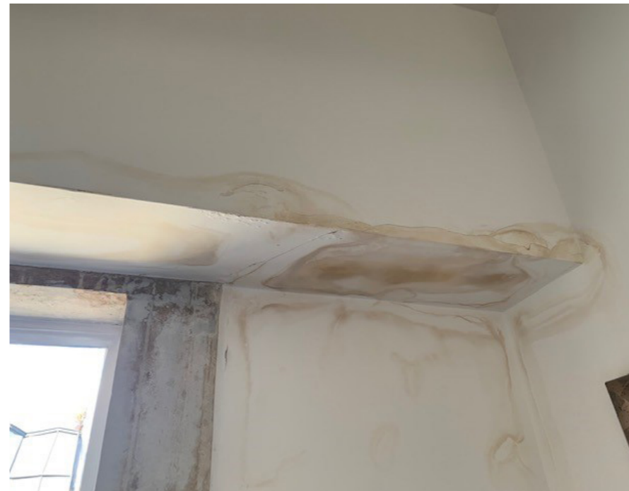
A photograph taken on the 01/08/2022 showing the existing internal condition and water damage to the first floor ceiling and original stone window surround.
