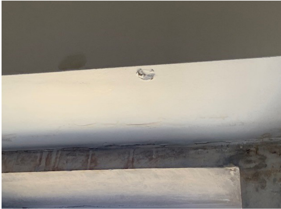
A photograph taken on the 01/08/2022 showing the existing internal condition and water damage to the first floor ceiling.
