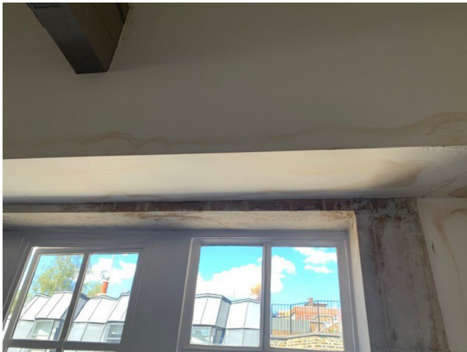
A photograph taken on the 01/08/2022 showing the existing internal condition and water damage to the first floor ceiling.
