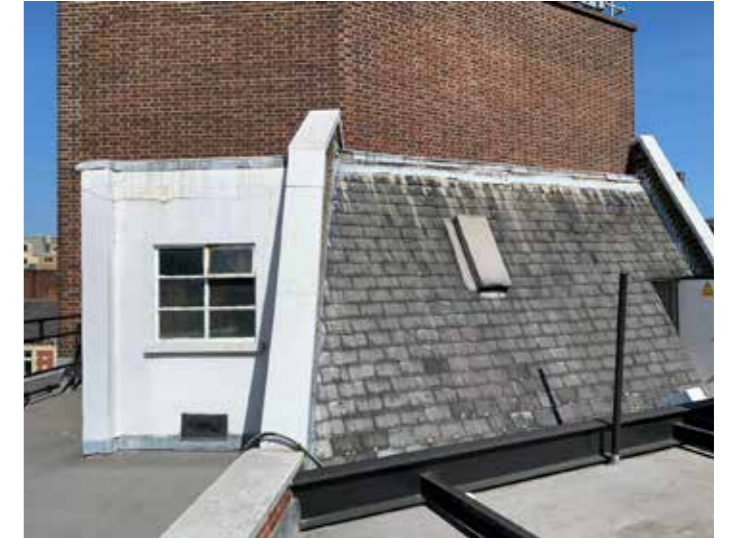
Figure 4.5 The roof is accessed by a small extension located in the north-west corner of the roof.
