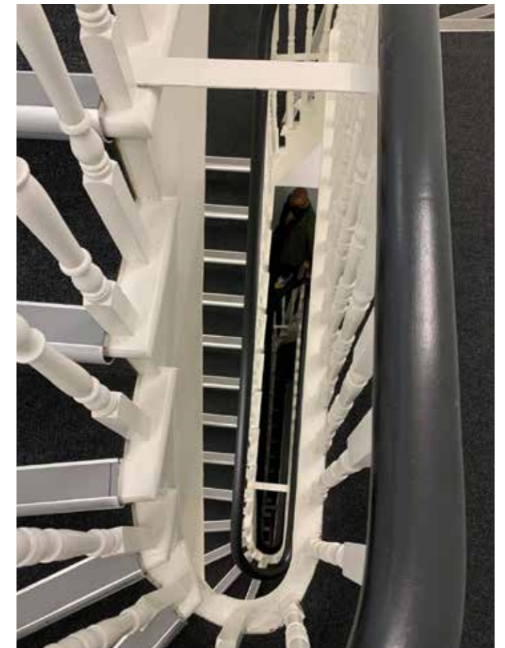
Figure 4.6 The staircase located in the north-west corner of the building has been extensively altered
