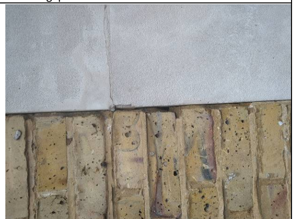
Photograph 12 – Concrete panel with minor gap along the edge where it met the brickwork on the wall of the property adjacent to the eastern boundary.
