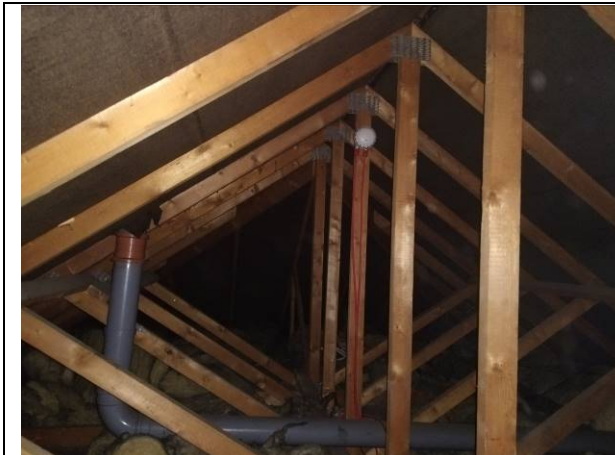
Photograph 7 – Enclosed roof void of Building B1 showing the bitumen felt under the tiles and cluttered space with numerous wooden joists.
