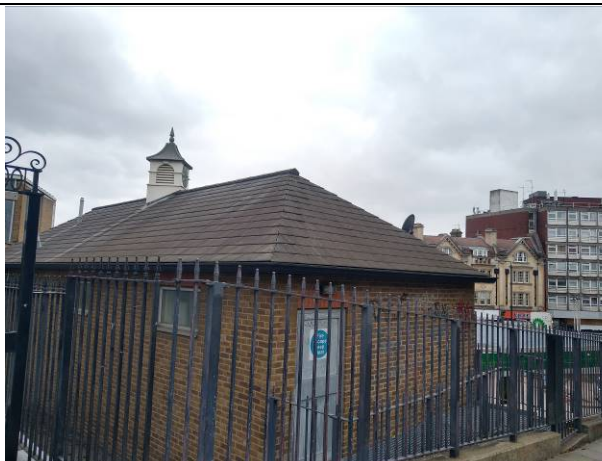
Photograph 5 – View of the hipped roof of Building B1 showing the close-fitting tiles and ornamental clock tower in the centre of the roof
