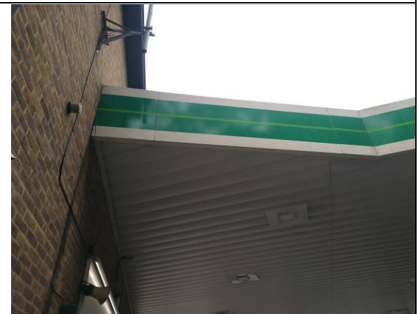
Photograph 10 – Metal panelling on the underside of Building B2's roof which was close fitting with no obvious gaps.
