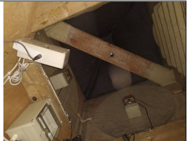
Photograph 8 – Inside view of the fibre-glass clock tower present on the roof of Building B1.
