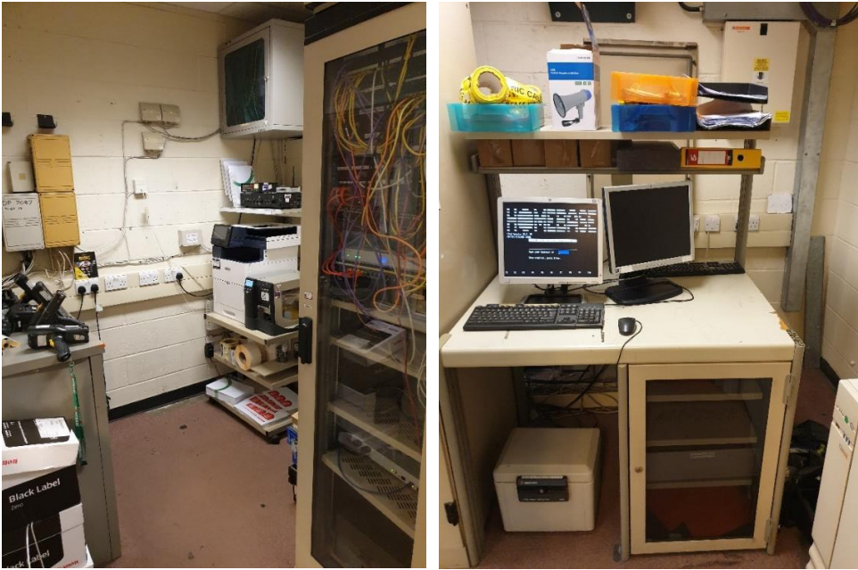
Figure 55 Potential WEEE from the operations room
