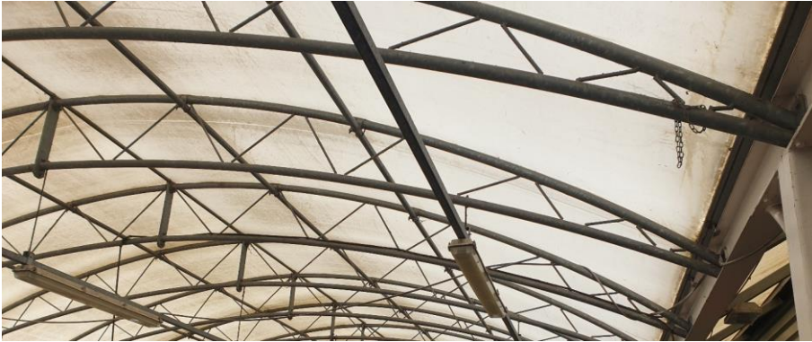
Figure 43 Garden area canopy – polycarbonate sheets
