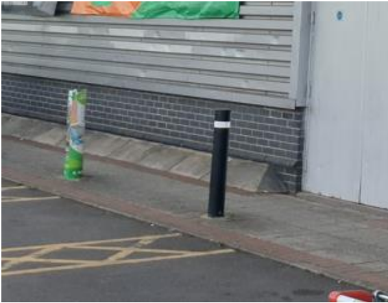
Figure 50 Bitumen close to the building
