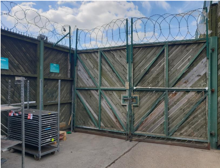
Figure 21 Posts, framing and razor wire fence
