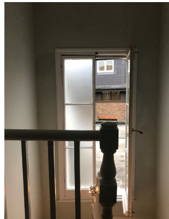
Figure 2E Single glazed doors onto flat roof area
