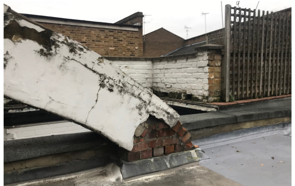
Figure 2I Cracked render and unstable bricks at base of chimney stack
