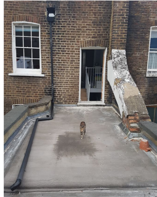
Figure 2G The flat roof area: evidence of standing water + unsafe chimney stack
