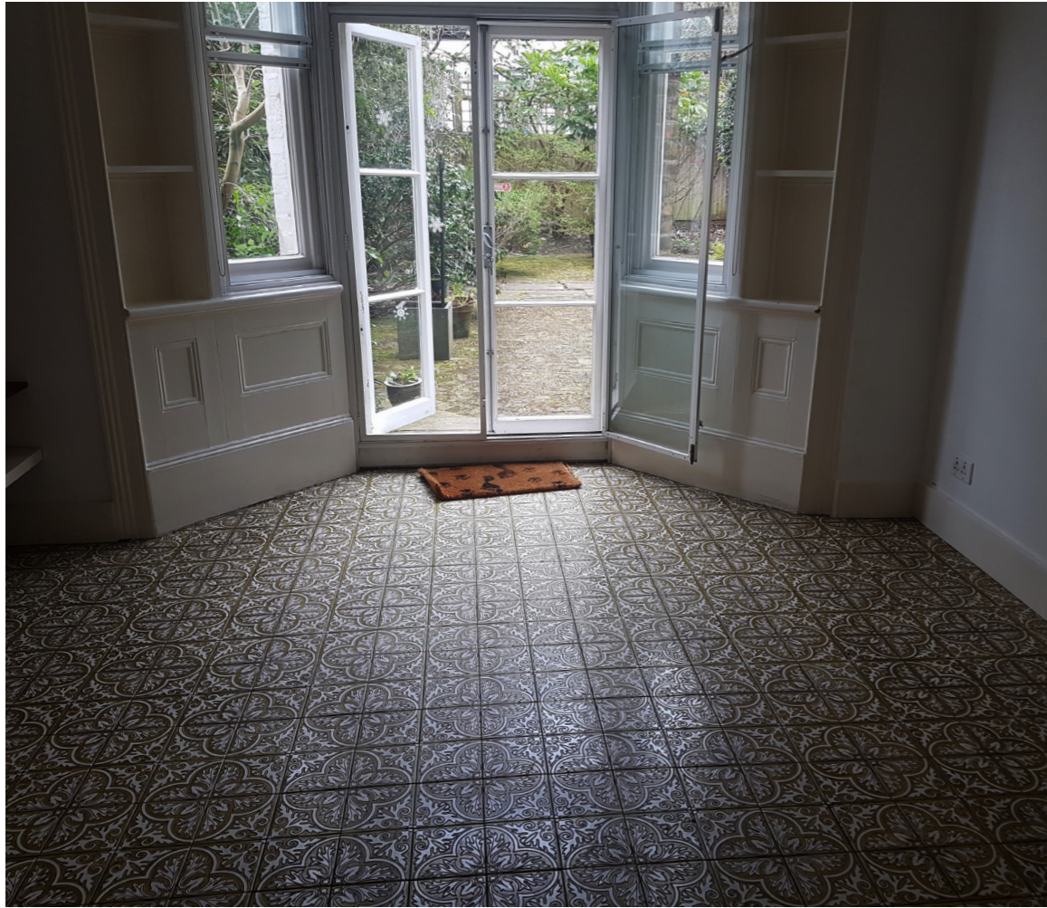
i) view of lower ground floor existing living room - poor internal light quality
