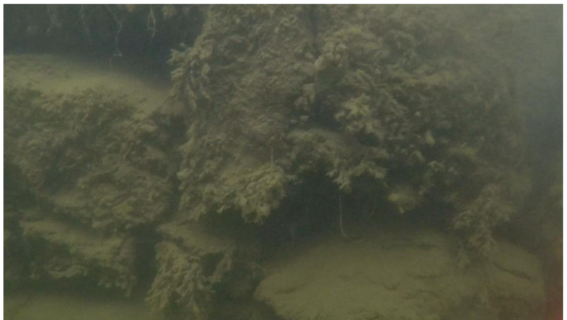
Figure 3.5: Typical gaps between blockwork due to mortar loss
