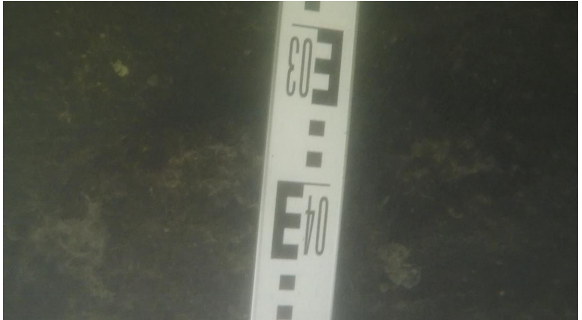
Figure 3.11: Image from video footage showing part of wall where the concrete layer is discontinued, and its thickness is reduced.
