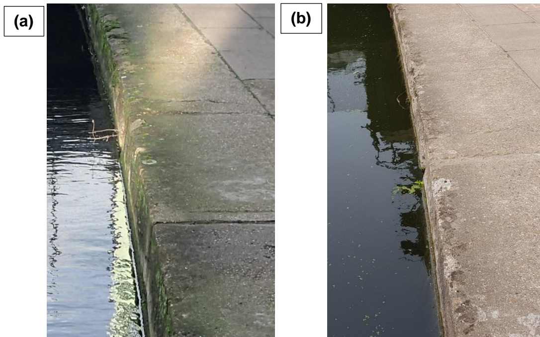
Figure 3.4: Extent of damage to capping beam edge observed during (a) 2019 initial inspection (b) 2022 reinspection
