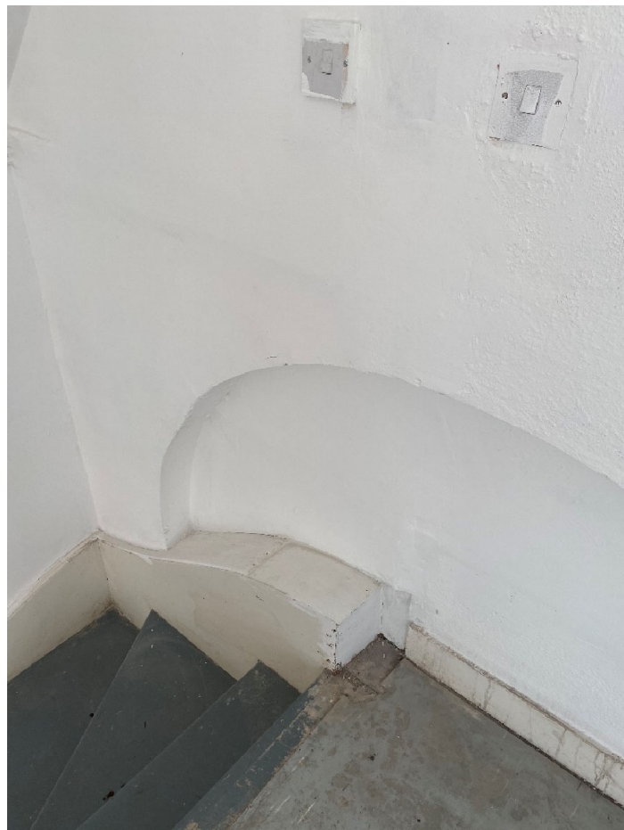
Figure 9. Modern stair crudely installed to cut across arched recess
