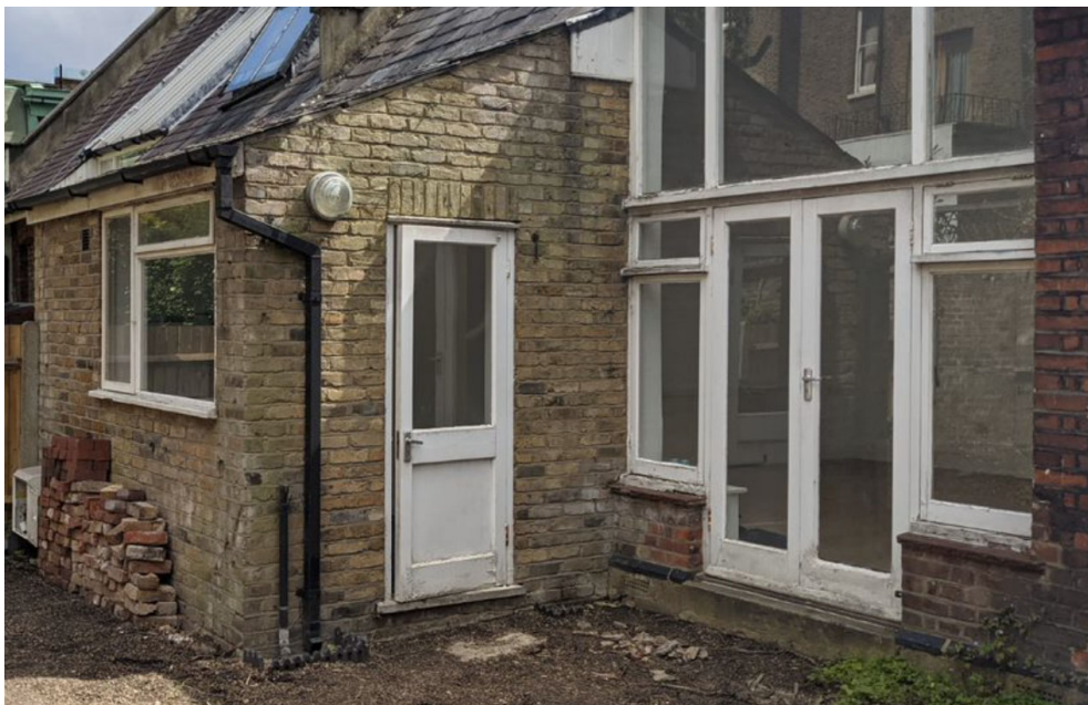
Figure 4: Studio 5 glazed screen as existing, along with assumed 1970s kitchen extension – a very different from to what was originally built.
