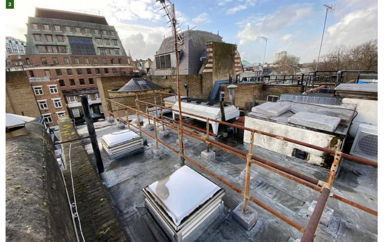
Figure 14. View from roof of 20-21 onto 22 showing typical roof plant, access and condition.
