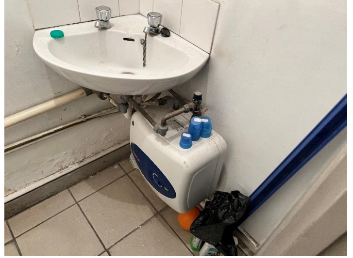
Sink in Toilet Ground Floor
