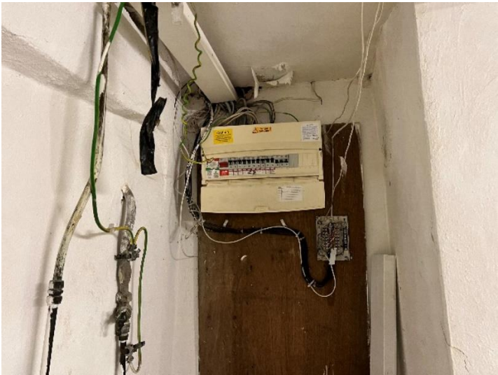
Mains electrical board- basement
