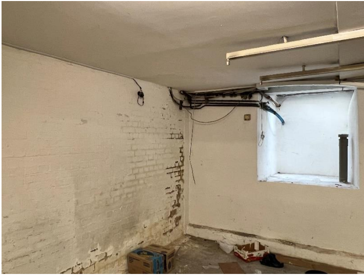
Basement- Incoming water pipe
