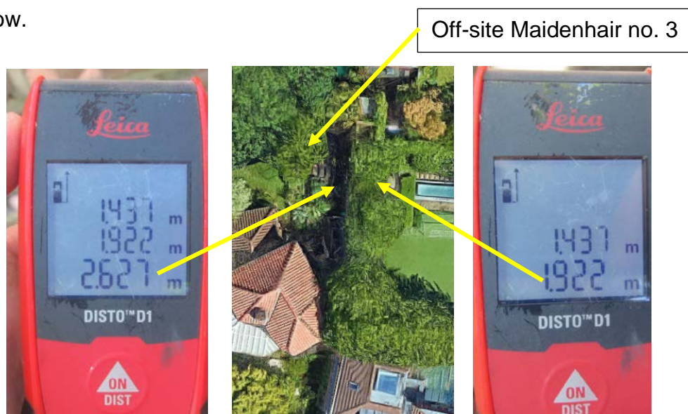
Images 3 – 5: Laser disto from top level of wooden palisade screening to existing ground levels on east and west side of boundary retaining wall
