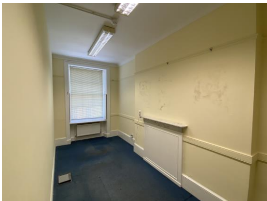
Figure 32: The surviving fire surround to the front of the 2 nd floor plan, now set within an incongruously proportioned room.
