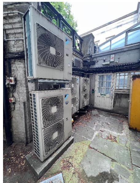
Figure 1—2 External plant area (view 2)
