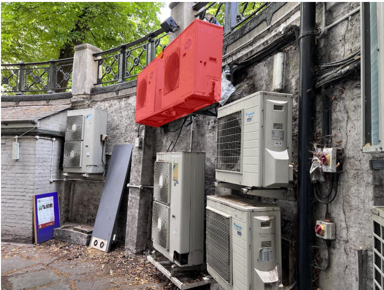
Figure 1—1 External plant area (view 1)
