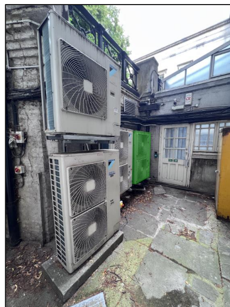
Figure 2—2 Operating condensers (view 2)
