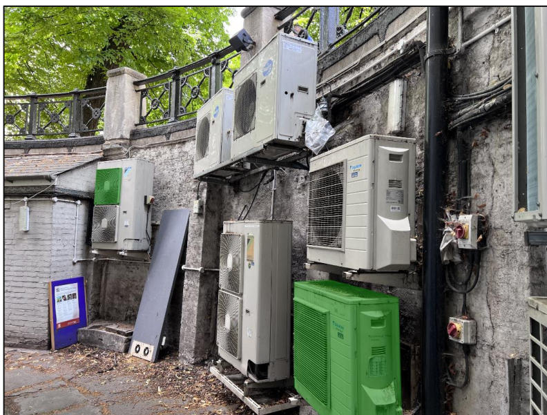
Figure 2—1 Operating condensers (view 1)
