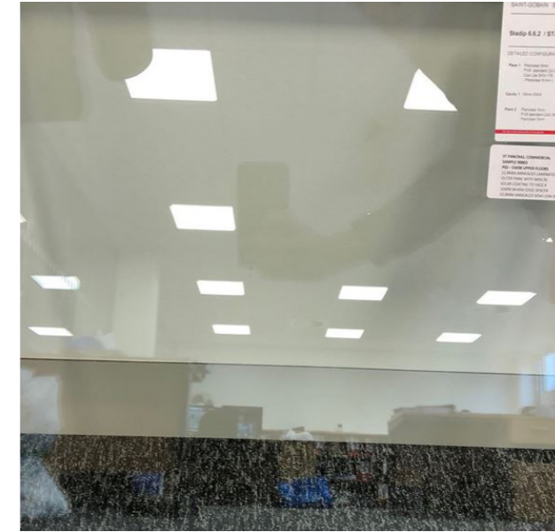
C7 - Glass Upper Material: Saint-Gobain glass, Pane 1; Planiclear (6 mm) PVB Standard (2 X 0,38 mm) Planiclear (6 mm) Cool-Lite Skn 176 Cavity; Argon (90%) / Air (10%) / 20 mm Pane 2; Planiclear (5 mm) PVB Standard (2 X 0,38 mm) Planiclear (5 mm)
