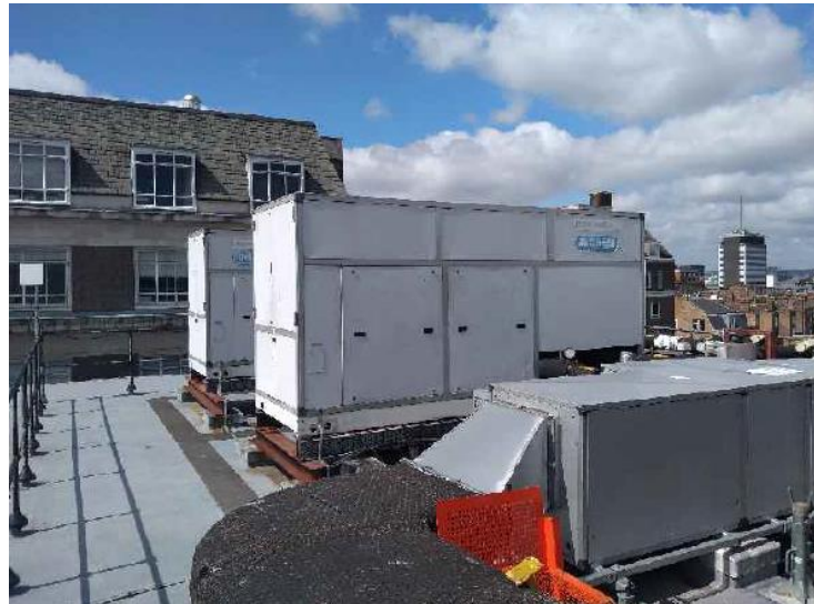
Figure 4: Existing chillers and air handling unit above 6th floor (to be removed)
