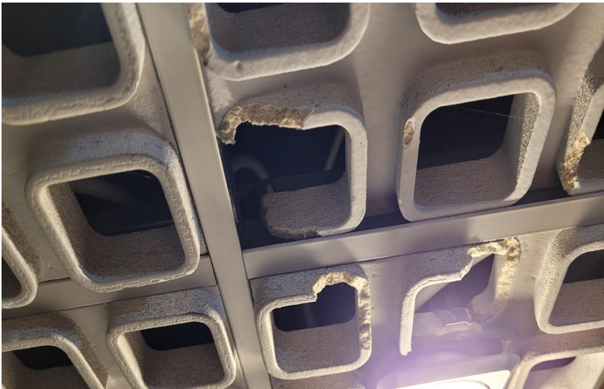
Photograph 4: Typical damage to suspended ceiling tiles in corridors and lobbies
