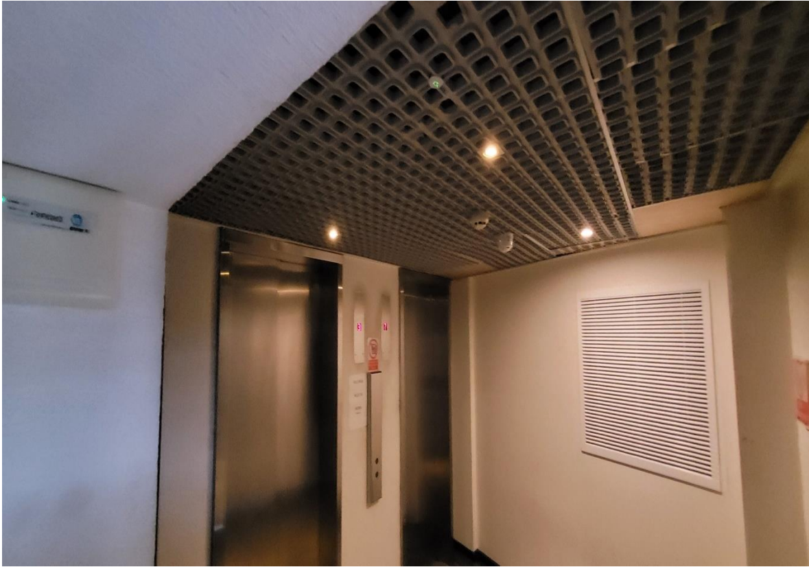
Photograph 1: Typical plywood sheeting to 3 rd floor lift lobby ceiling where ceiling tiles missing
