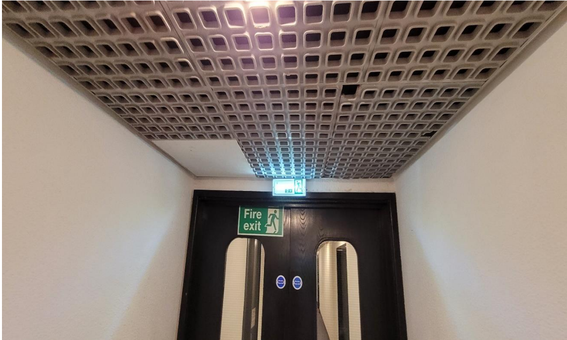
Photograph 5: Typical damage to suspended ceiling tiles and non-matching tiles where ceiling tiles missing in corridors
