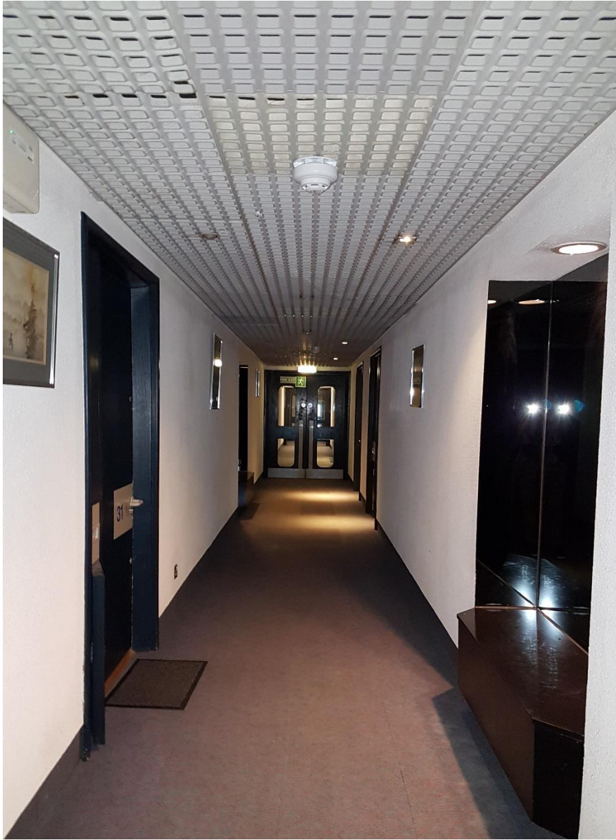
Photograph 7: Typical view of suspended ceiling and inadequate lighting to corridors
