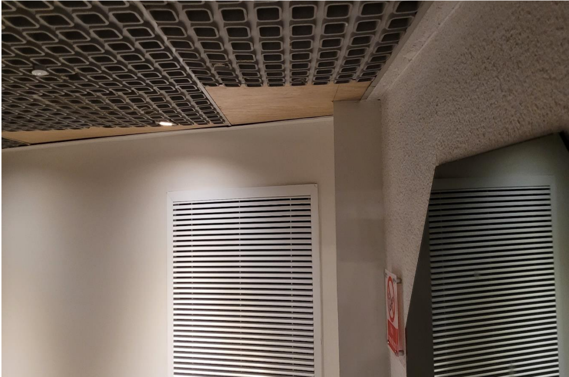
Photograph 3: Typical plywood sheeting to 5 th floor lift lobby ceiling where ceiling tiles missing
