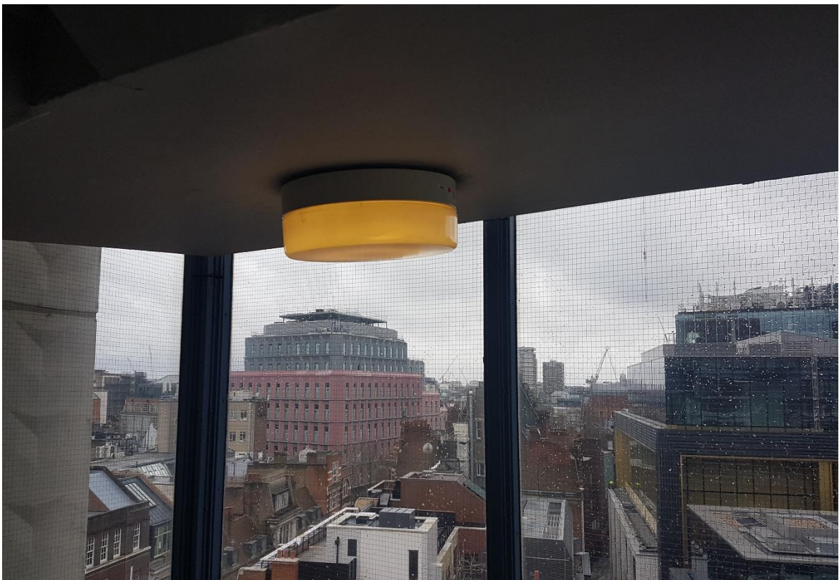
Photograph 9: Example of existing 2D bulkhead light fitting throughout staircases
