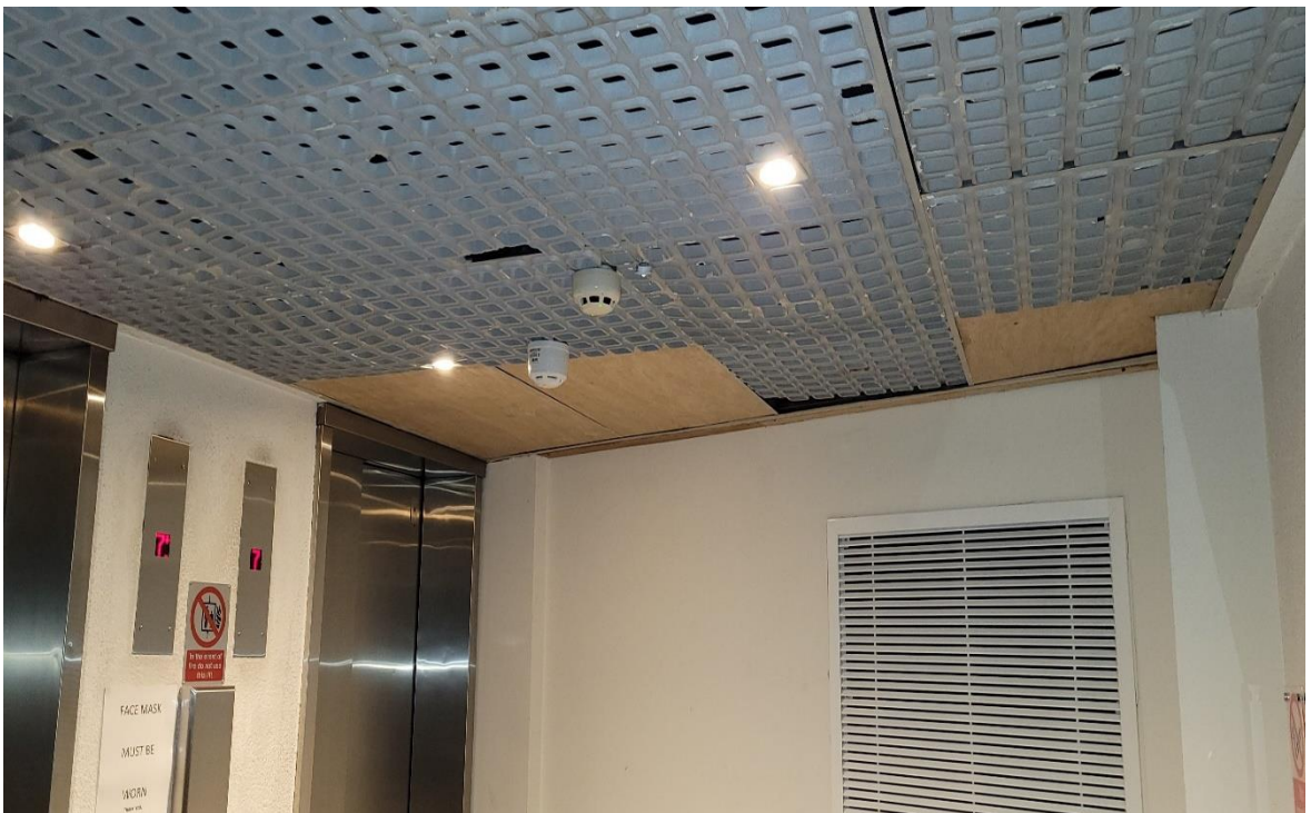
Photograph 2: Typical plywood sheeting to 7 th floor lift lobby ceiling where ceiling tiles missing
