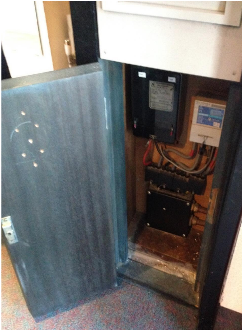
Photograph 11: Electric meter situated inside the cupboard that forms part of the apartment front entrance doorset.
