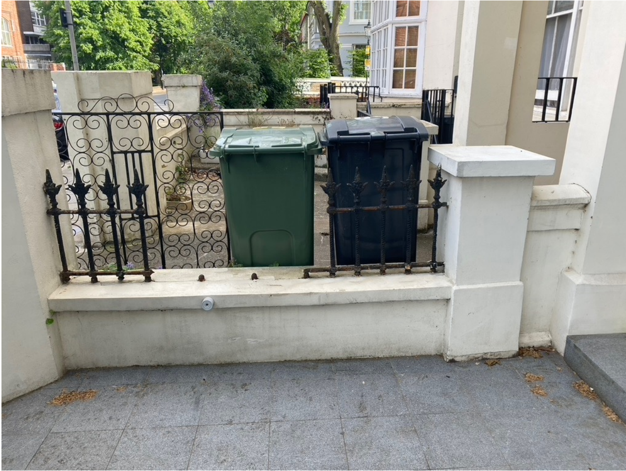
Railing between 61 and 59 that has been broken for 20 years that photographic evidence shows cannot be original
