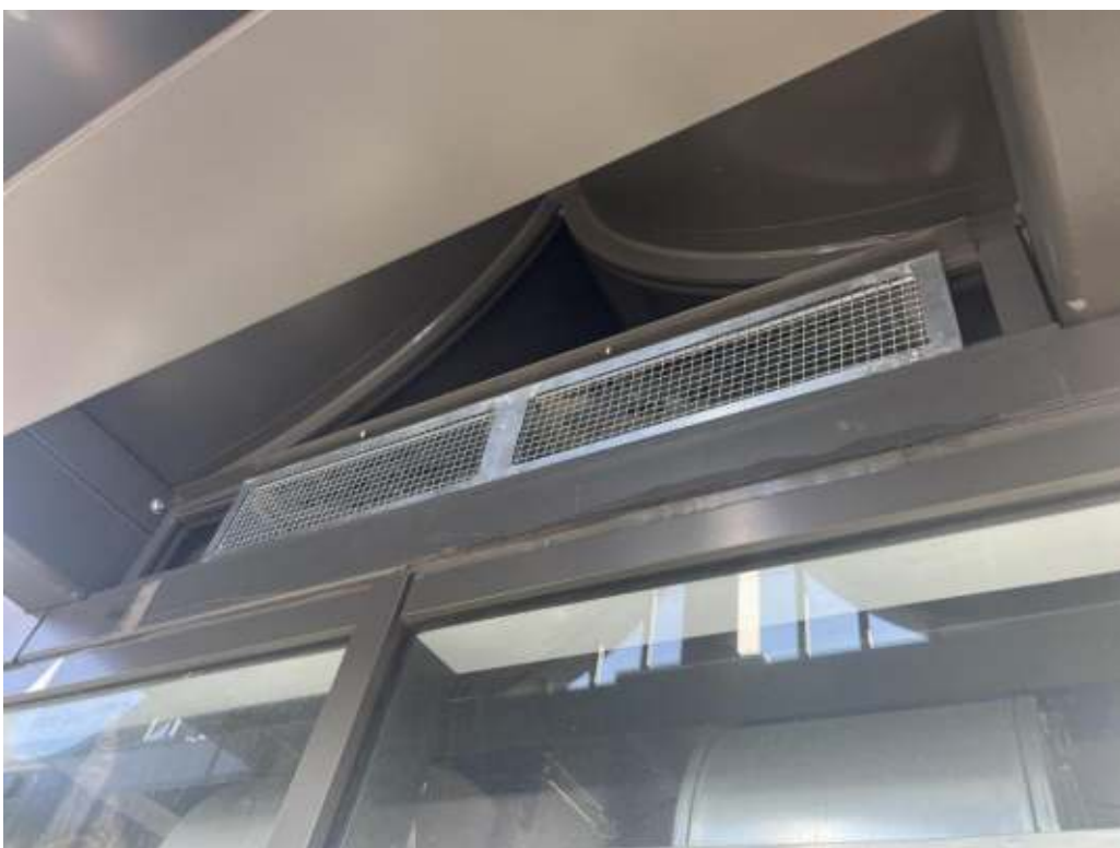
Figure 4: Extract louvres, atmosphere side
