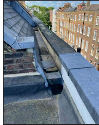
Fig. 6 - Existing shared outlet
