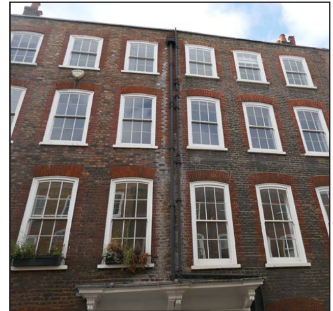
Fig. 9 - Existing stained brickwork to be cleaned and repaired
