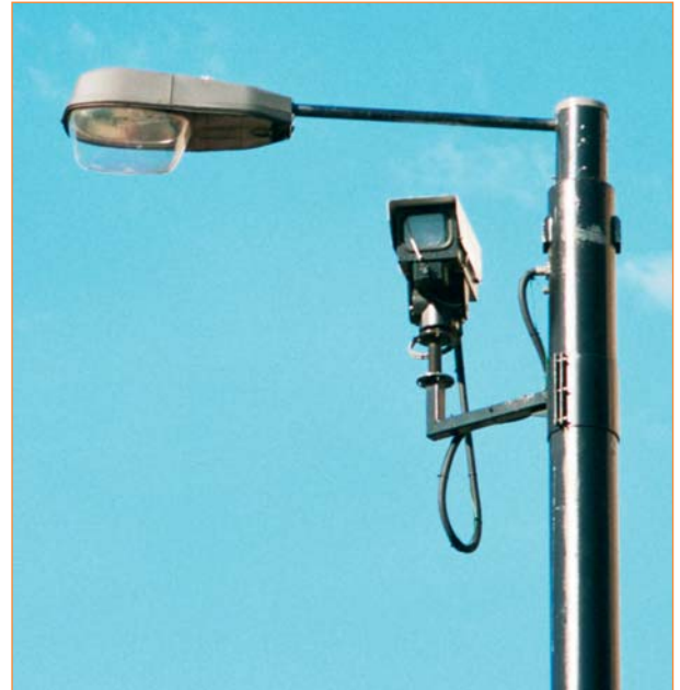
Combined CCTV and lighting column
