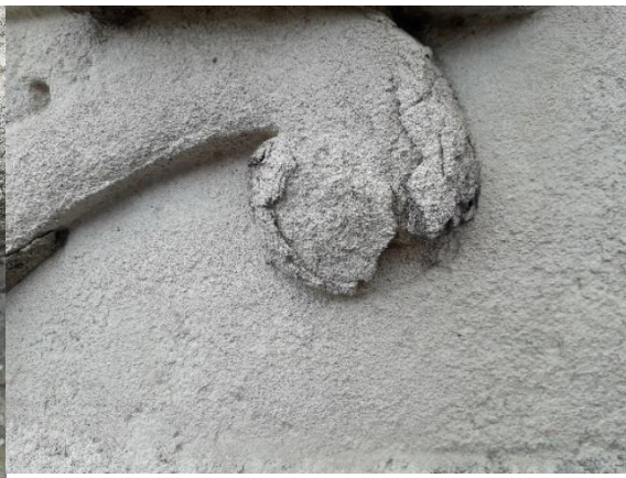
Figure 28 Smaller scale losses due to flaking/ delamination
