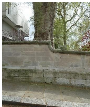
Figure 22 Southern boundary wall cracked and distorted by the growth of the tree and the displacement of the wall westwards towards gate pier 1.
