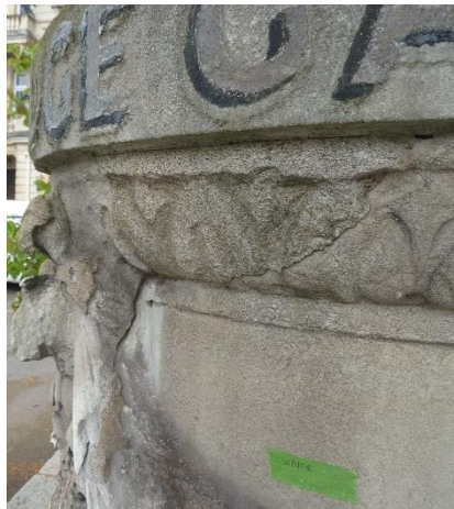
Figure 38 MP1, cyma still readable. Large repair to one area approximately 20cm
