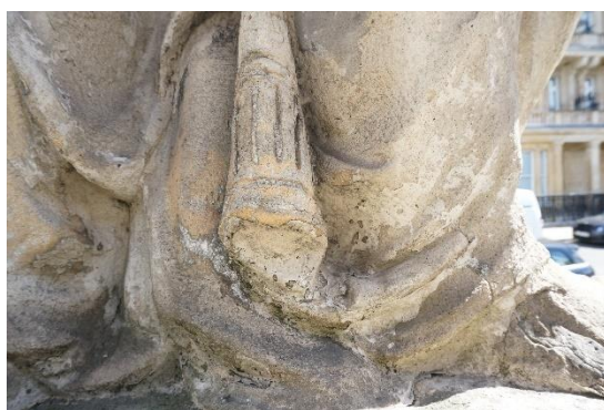
Figure 86 Paint clogging the detail
