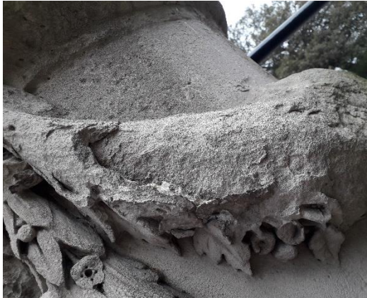
Figure 25 Sudden loss of large areas of detail from deep cracks within the stone
