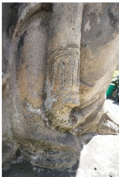
Figure 76 MS4 Yellow staining of unknown cause
