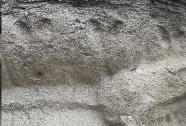
Figure 26 Surface erosion with gradual but almost total loss of detail and softening of carved edges. These areas are clean where the water has washed the polluted surface away
