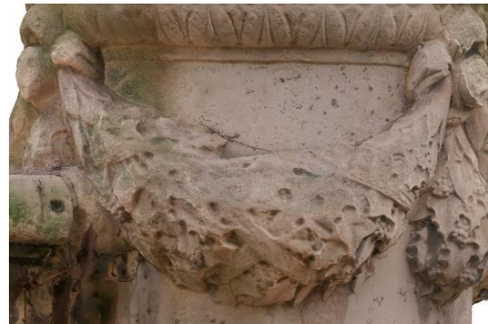
Figure 34 MP4 moderate erosion to detail, cyma detail can be read
