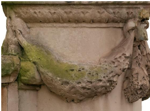
Figure 33 MP1 moderate to bad erosion. Swags eroded badly on two sides of the plinth. Cyma pattern is almost discernable but worn.
