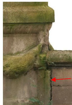
Figure 23 Wall-plinth joint south side. Historic fill and continued movement with a 3mm gap and southward displacement
