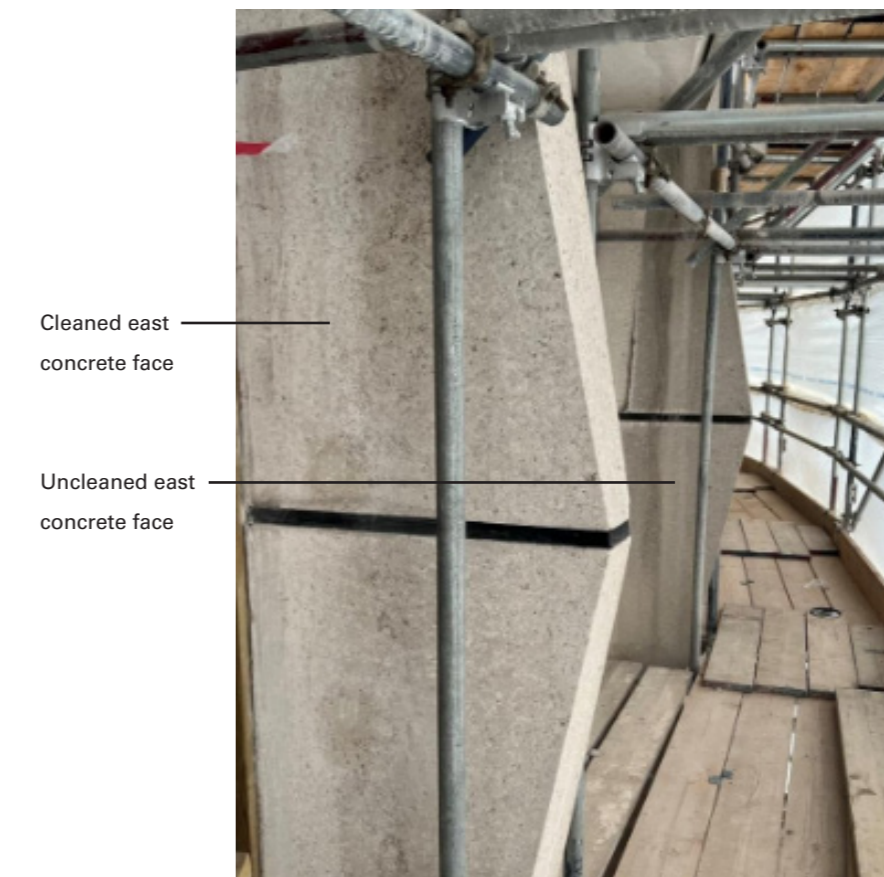
Fig. 2.1.5 East concrete faces (cleaned and uncleaned)
