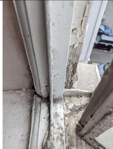
Existing window frame & joint_ weathered and damaged
