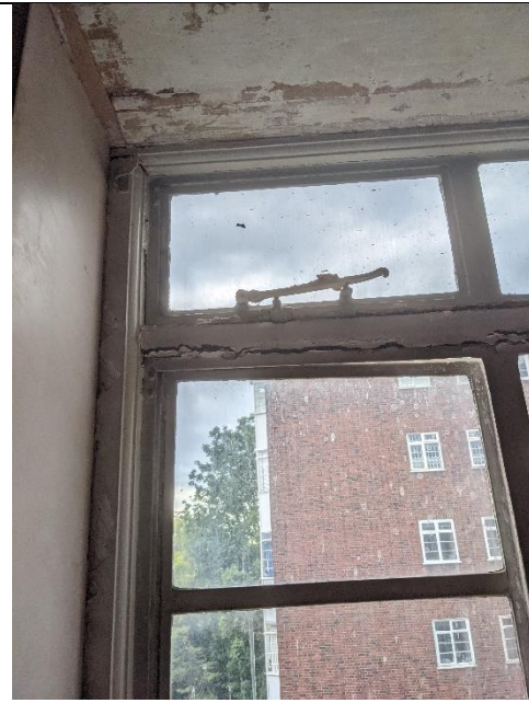
Existing window frame_ Cracked
