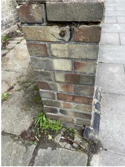
Image 1 – fixings of old metal gate
