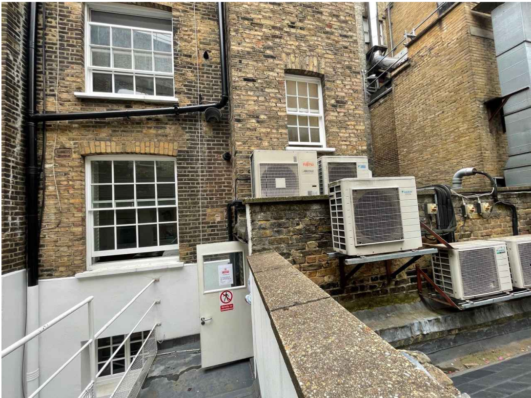
Photos of the air conditioning units
