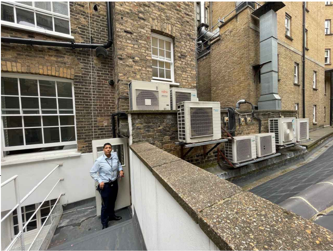
Photos of the air conditioning units
