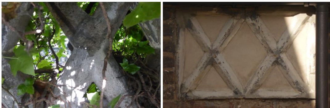
Figs. 5,6 Number 22 Gloucester Crescent – the immediate neighbour to the proposed site with dense ivy covering the original 'saltire' wall panel – note fractured surface revealing corroded iron reinforcement – Fig. 5 shows a pair of original 'saltire' blocks visible on the party wall to number 23 Gloucester Crescent itself.
