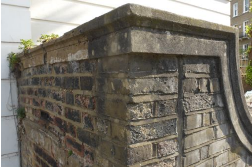
Fig. 8 Number 23 Gloucester Crescent return party wall – note original section of buff coloured Roman cement coping and junction with new corner moulding in grey Portland cement with rebuilt corner in modern bricks with weather struck cement pointing.
