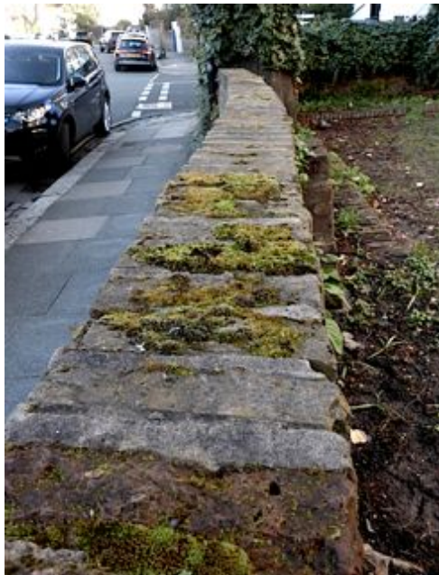
Fig.8 Detail of West wall cement mortar bedded coping using a soldier course
