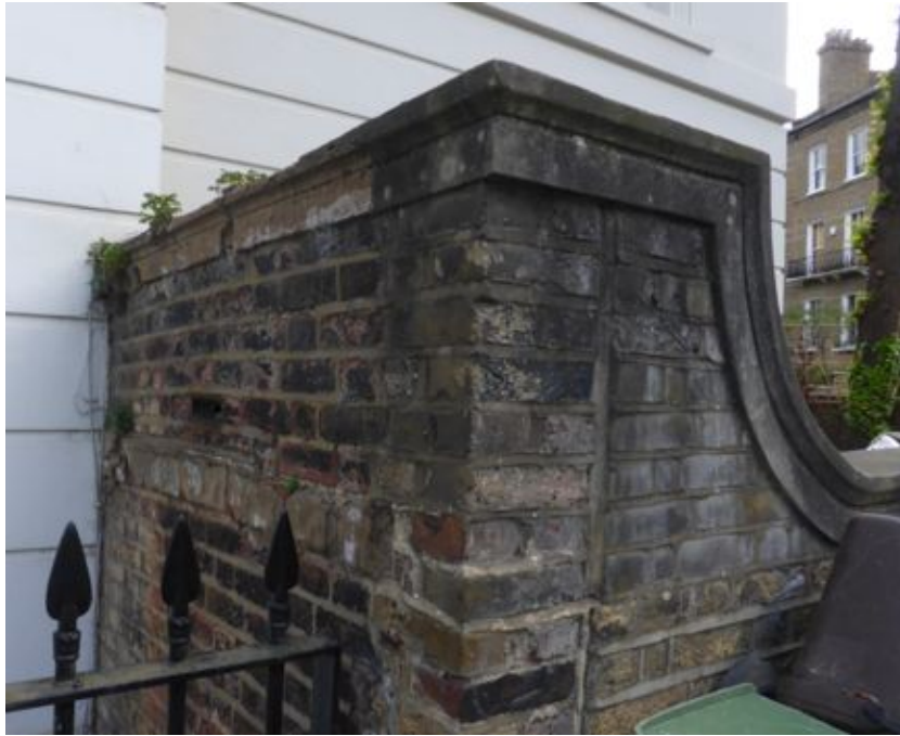
Fig.5 Corner detail showing original Roman cement coping and band which frame the dimension of the 'saltaire' blockwork.
