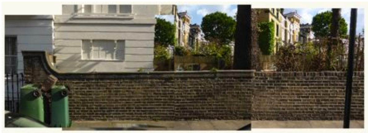
Fig.4 Composite photograph of the North boundary wall, rising with a swept coping detail to the original wall height.
