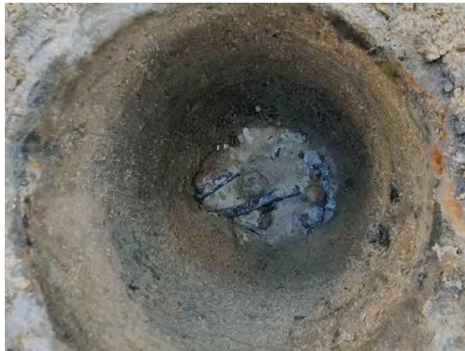
BH01 core broken out 01/11/21 with rebar at 600mm bgl
