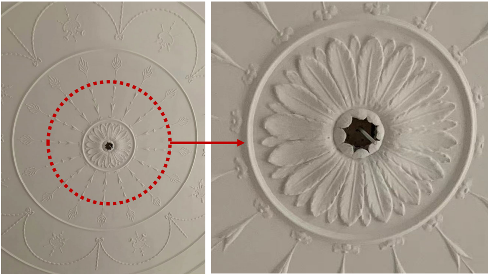
1 st Floor Reception Ceiling Rose
