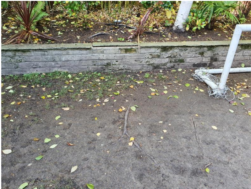
Photo 11 - birch roots visible within lawn area:
